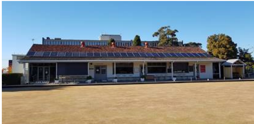
Photo: Solar panels on the Footscray Drill Hall
